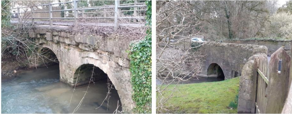
L: Bridge over By Brook. R: Bridge over Box Mill tail race. Photos Varian Tye
